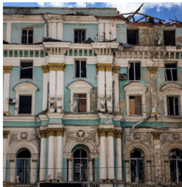
Fig 4. A damaged building in Kharkiv, 23 May 2022. © Dimitar Dilhoff/AFP via Getty images.
